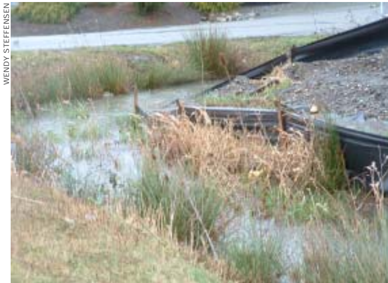
This poorly maintained silt fence is collapsing, allowing sediment to get into a roadside ditch that leads to a creek.
