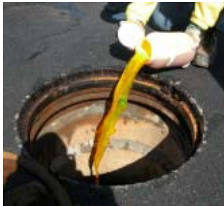
Fluorescent dye is poured into a septic tank that may be failing.
