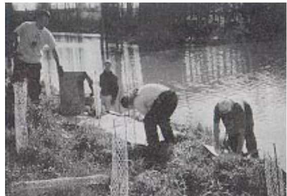
CRUE students work on a restoration site. Newly installed plants are surrounded by mesh tubes for protection from predators.
