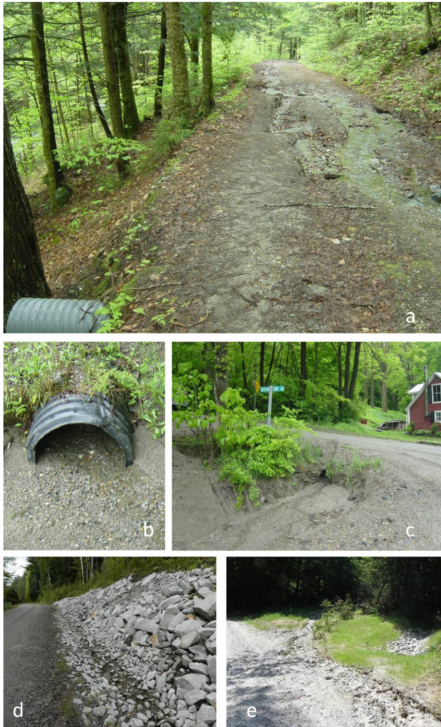
Figure 1. Examples of erosional and depositional features on roadways that impair water quality, including (a) fluvial erosion of road surface, (b) plugged culvert, and (c) slump on roadside margin. Also shown are examples of best management practices used to address water-quality impairment from roads, including (d) a stone-lined ditch designed to reduce erosion of roadside ditch and cutslope and (e) turnouts used to divert eroded sediment into roadside forest and away from receiving waterways. [Colour figure can be viewed at wileyonlinelibrary.com ]
