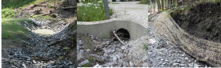
Figure 10: Examples of assessed BMPs—left: intact stone lined ditch; middle: culvert compromised by debris partly plugging inlet; right: failed BMP installation showing evidence that stone and stabilization fabric have been undermined.
