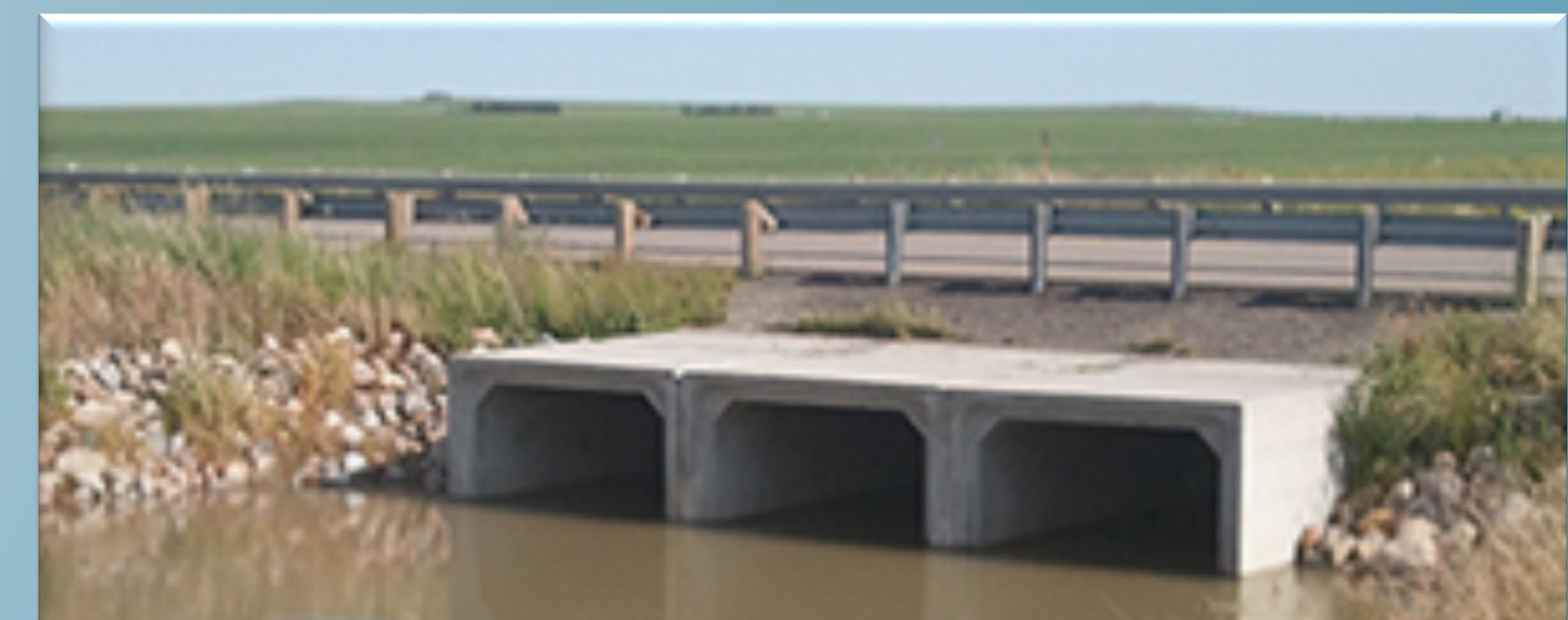
Figure 3. A culvert constructed under a road with a minimal barrier wall. Barrier walls for this study would be taller and more solid. Photo from Roseke Engineering.
