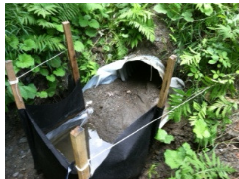
Figure 2: Plastic and filter fabric silt fence, installed out culvert outfall, with bulk sample collected after storm event in summer 2012
